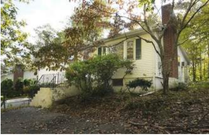
A house at 857 Grove St. Terrace in Worcester is contaminated with mold. (T&G Staff/RICK CINCLAIR)
