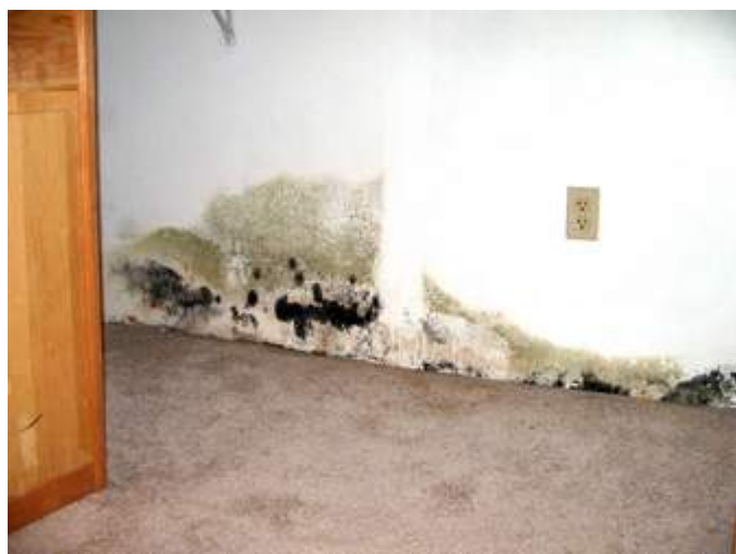
Mold creeps up the wall of this basement. (PHOTO COURTESY OF JASON MERCER)
